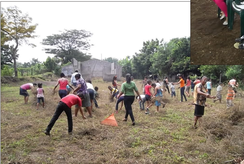
Children are helping to clean the property in Telica where a church is being built.
